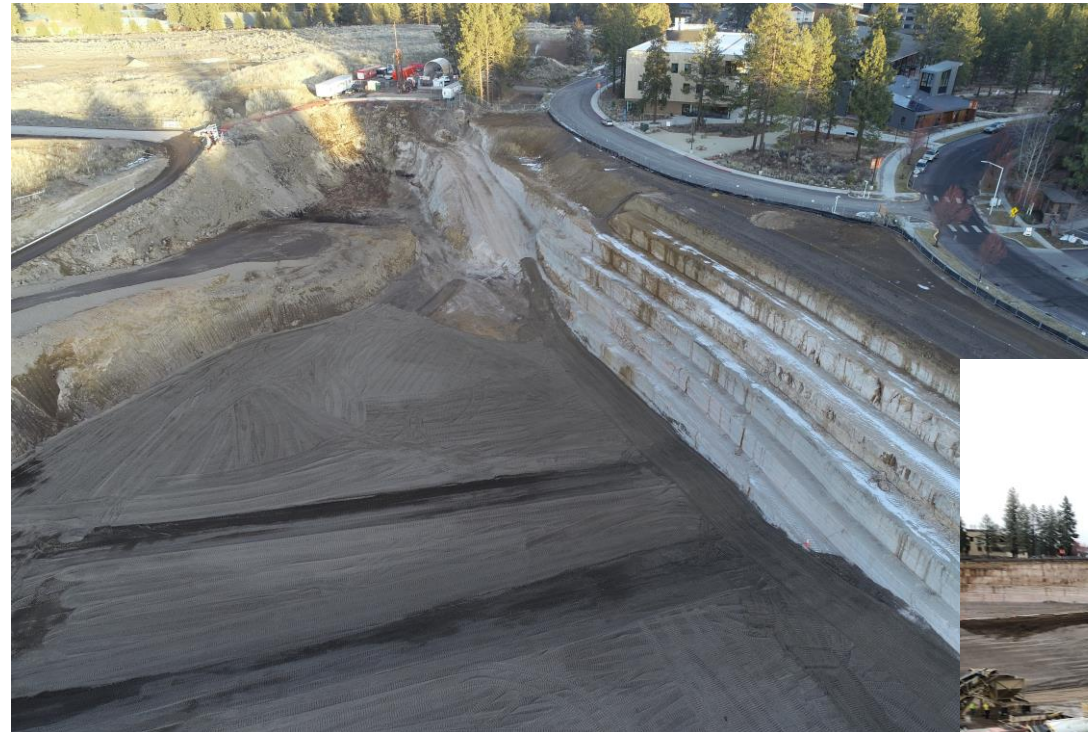
Aerial View of South Side of Pit benching and filling pit floor activities
