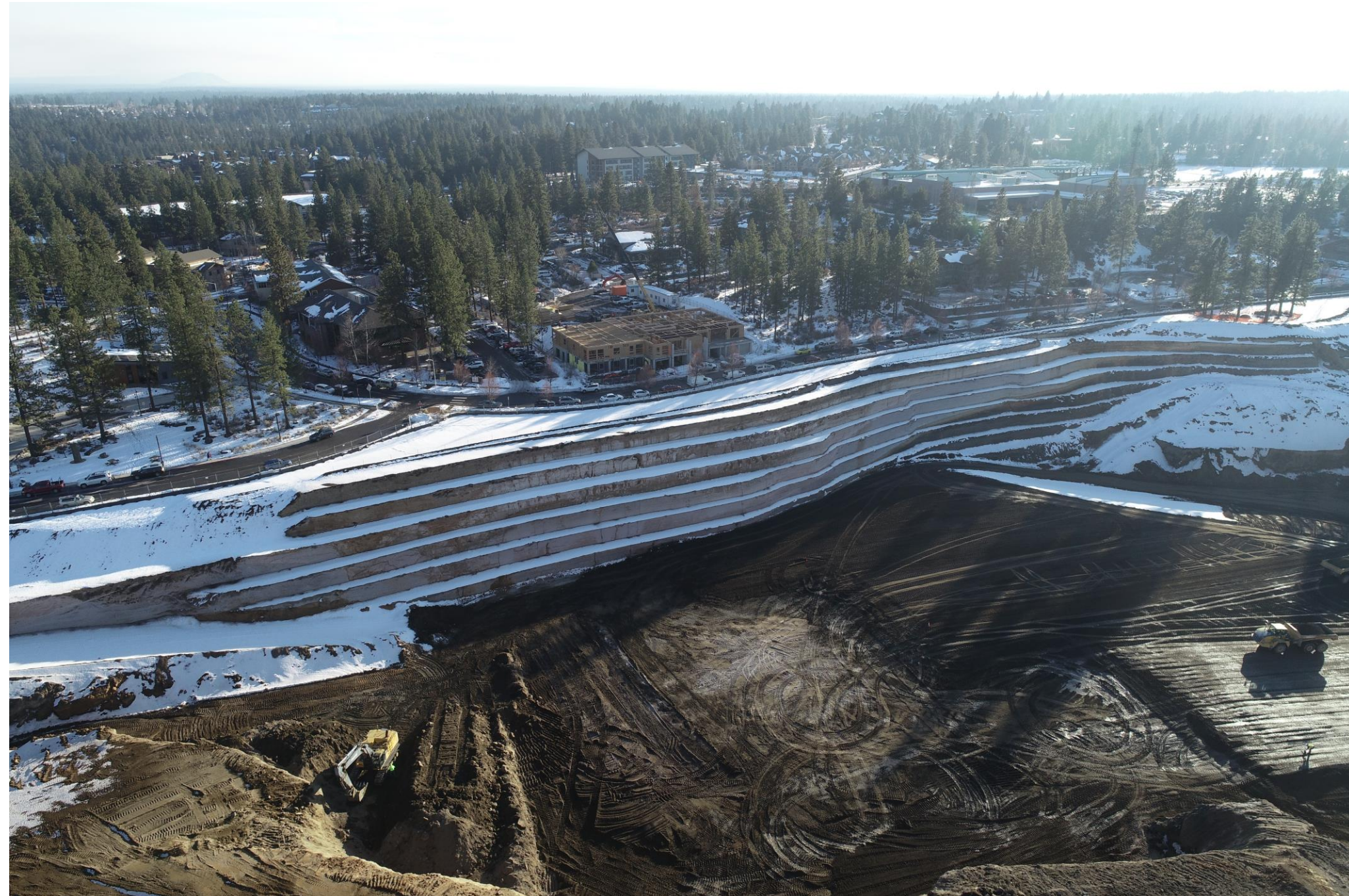
Aerial views of the south benching of the pit and ongoing grading activities of the pit floor
