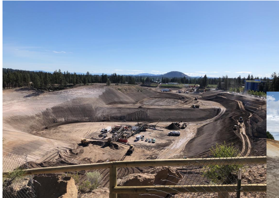
View of the pit from the west cliff wall – crushing, split rail fence, and embanking activities on the south side of the pit
